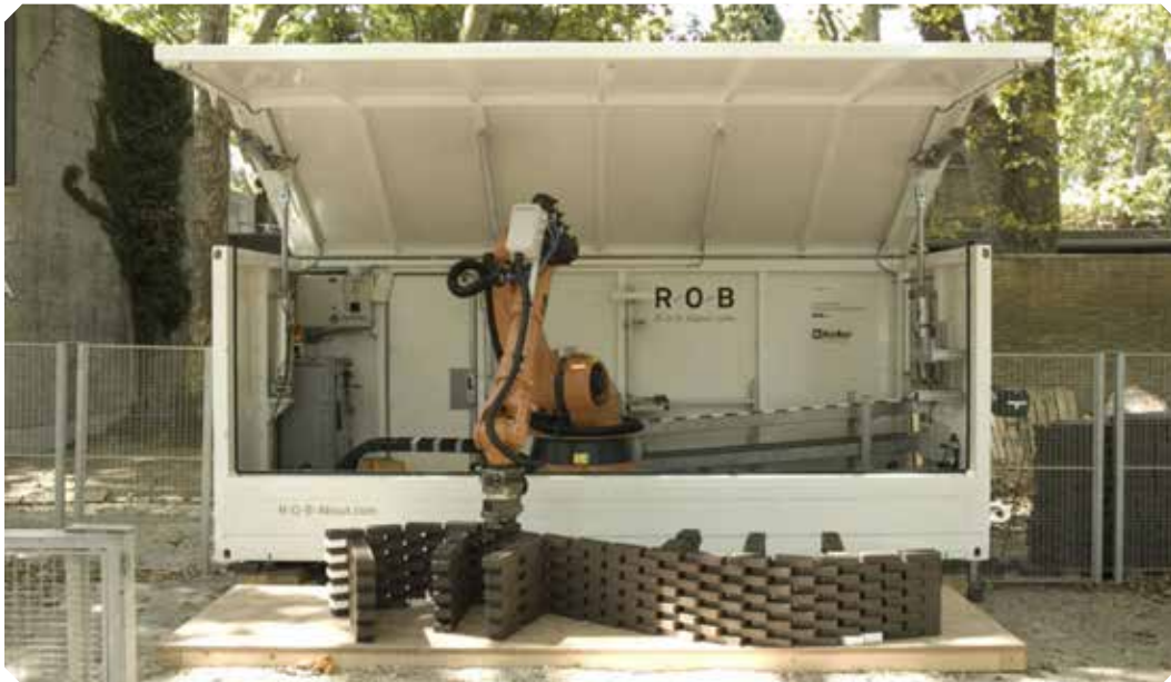
Fig. 1.2. The ROB unit building a section of Structural Oscillations. The deployable unit performs meticulously pre-calculated onsite fabrication. (Gramazio & Kohler © ETH).
